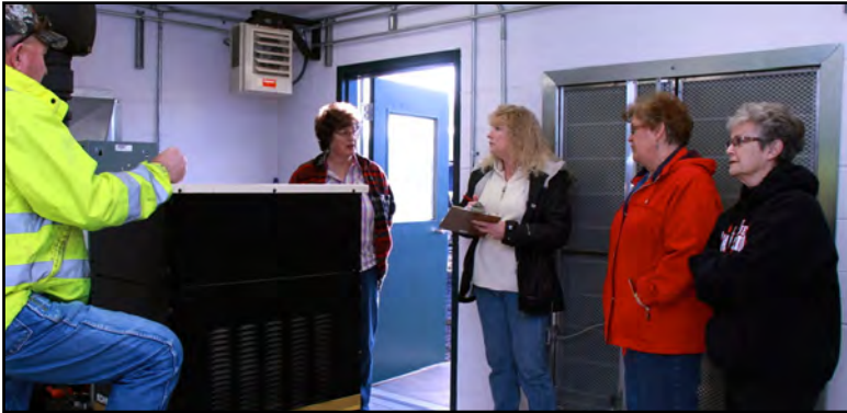
Contractor Mike Becker talks about the lift station generator with Donna Neumann, Engineer Becky Sheridan, Linda Kerr and Louise McKinnon.
